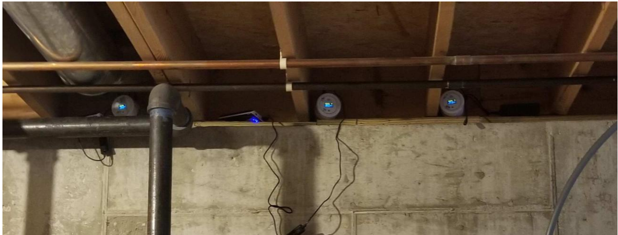
Figure 24: EcoTrackers placed in a basement near adjoining slab
